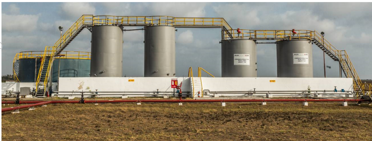
Bhandut Processing Facilities
