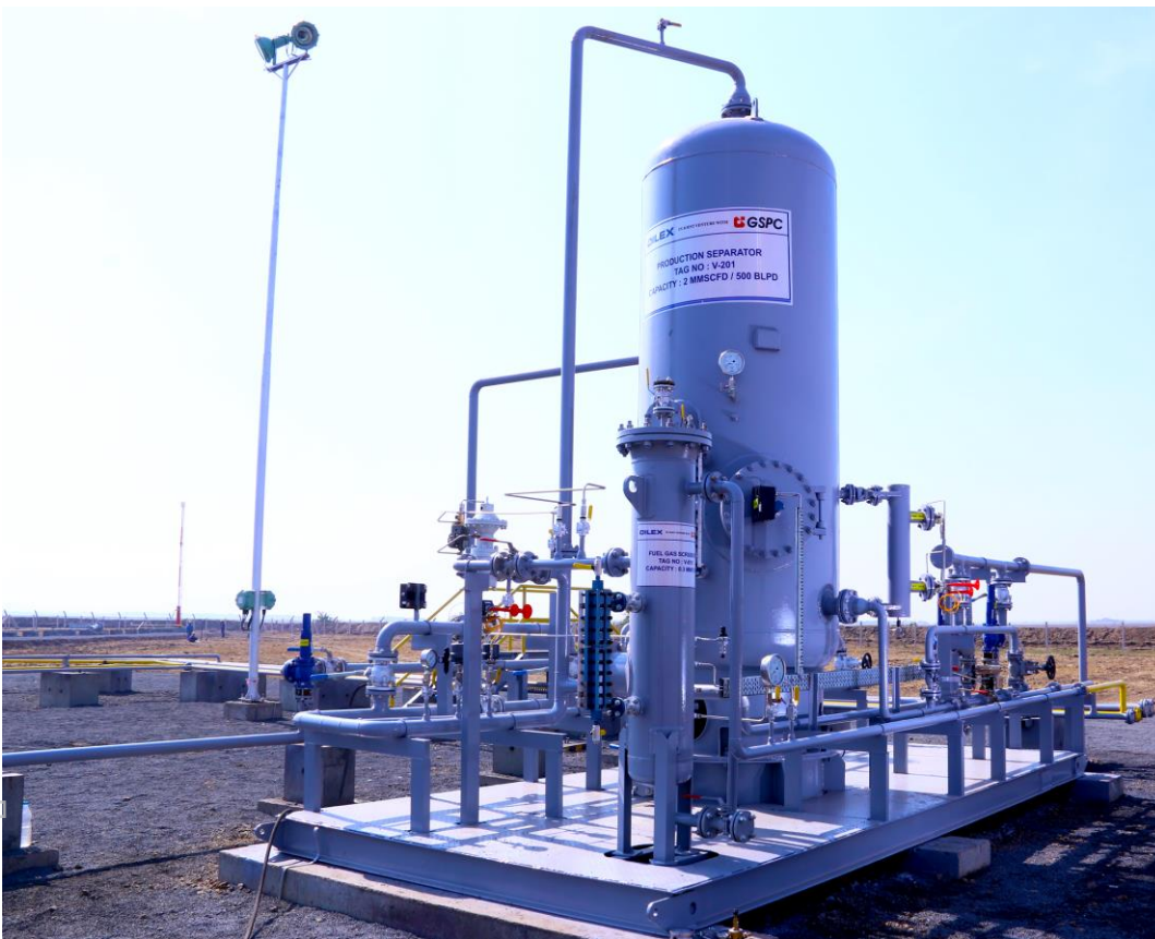
Figure 2 Separator, Bhandut Facility
