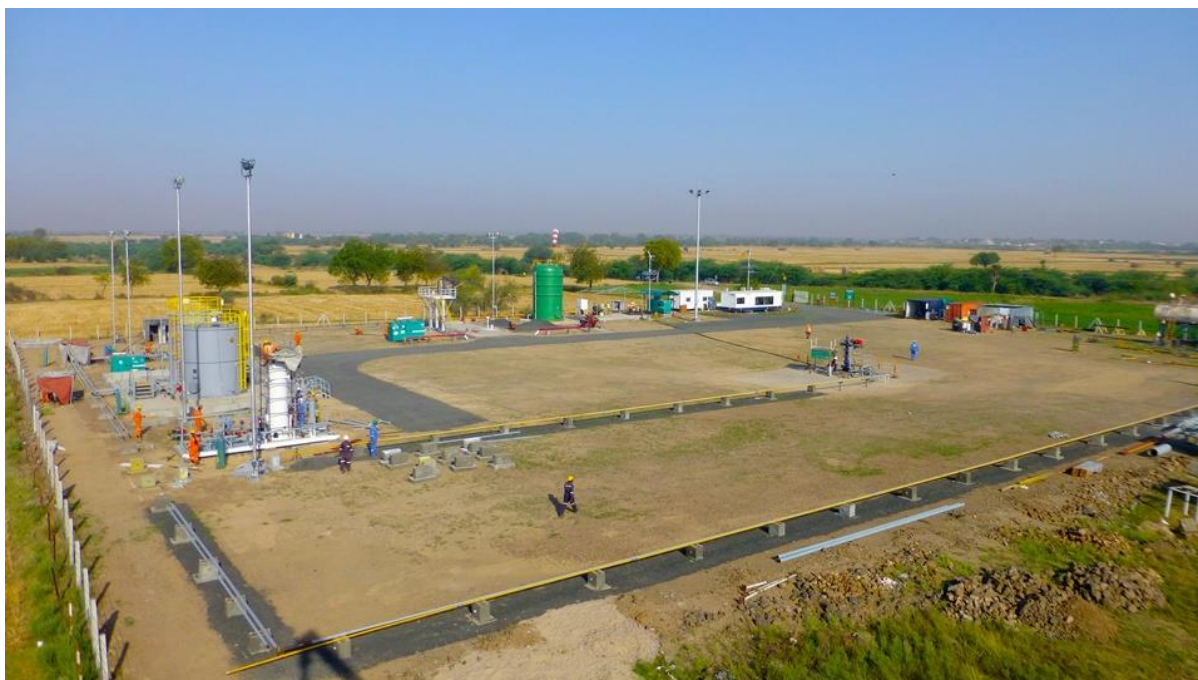
Cambay-73 production facilities
