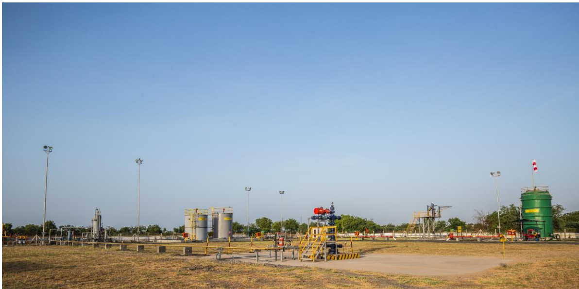
Figure 4: Cambay-73 Production Facility
